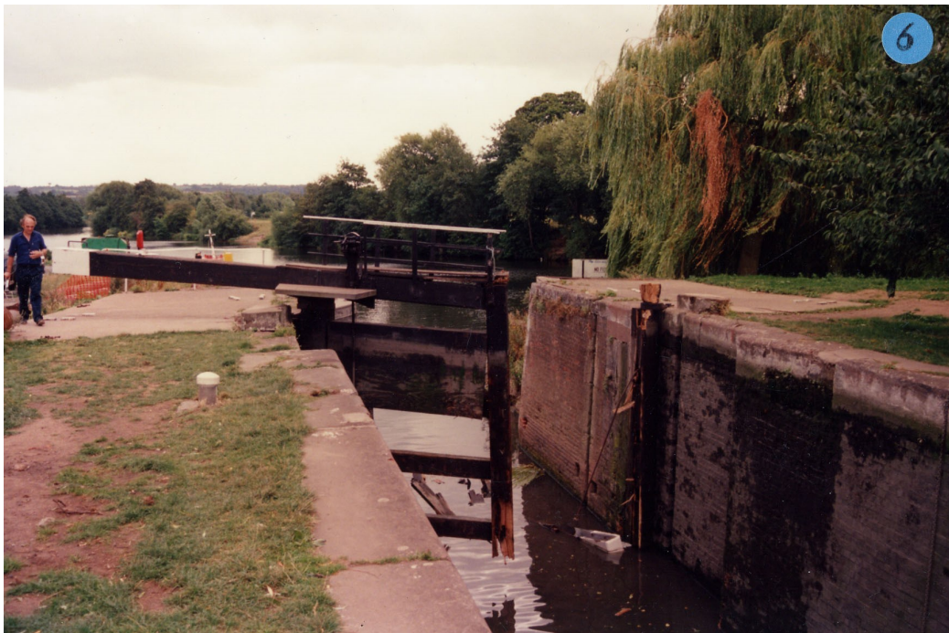
Nos 1 Broad Lock damaged by a hopper crash in 1980's
